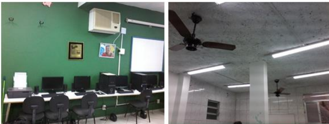
Picture 2 - Window Air Conditioner and Communication networks (left); Ventilation and illumination supplies (right)
