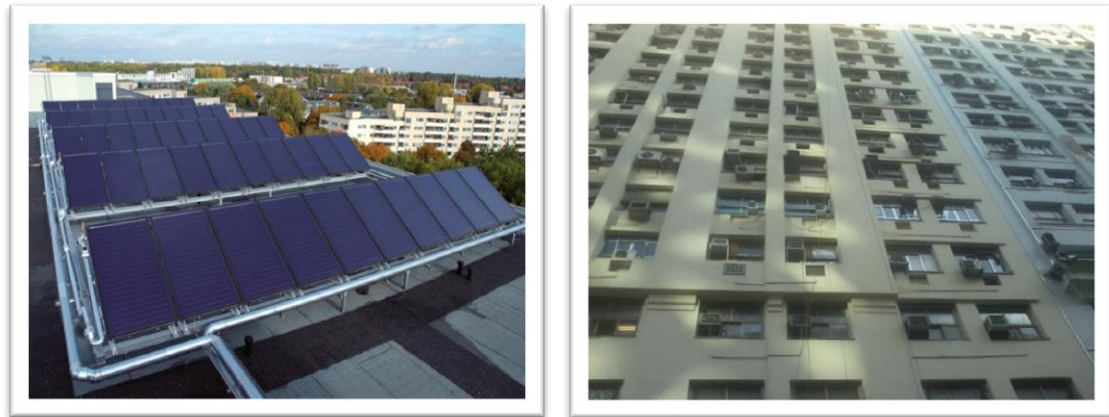
Figure 2 - Thermal Solar Array and Figure 3 Split Coolers with Compressor Operation
